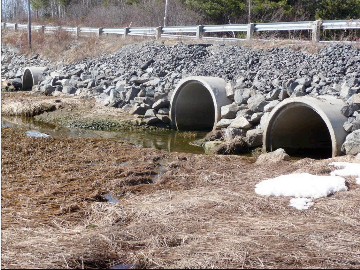
Figure 6 The three culverts installed at SG in 2006 (Upstream). Photograph by T. Bowron, 11 March 2010.
